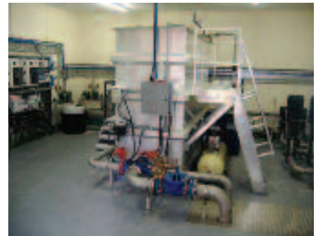
Castlebaldwin WTP, Co. Sligo
