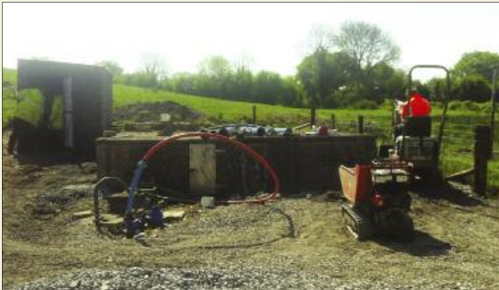
Improvement works are underway at the spring source supplying Clareen GWS in County Offaly.
