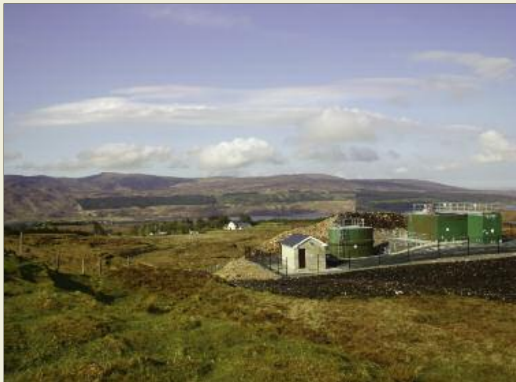
Perched in an upland area on the lower slopes of Errigal mountain, the recently-completed water treatment plant supplying Meenabool GWS in Co. Donegal includes sand filtration and chlorine disinfection. In an area of outstanding natural beauty, camouflaging has been used to ensure that the structures aren't visible from a distance.
