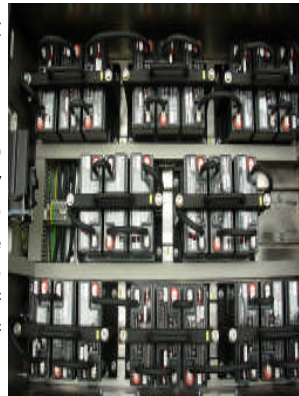
Pitch control battery (assembly of 144 battery cells of 2V/16Ah each)
