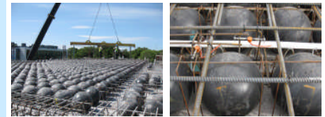
Figure 4: 'Cobiax' void-form flat slab system being installed in the NEB (left) and with gauges installed (right).
